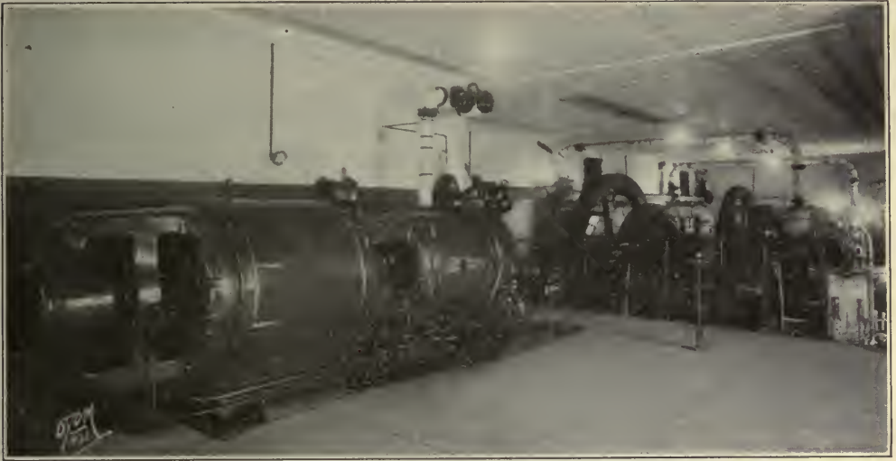
INTERIOR OF POWER-PLANT OF THE GREENVILLE, TEXAS, LIGHT AND WATER WORKS
